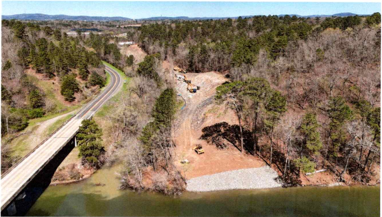
Davidson Drive WWTP Discharge
