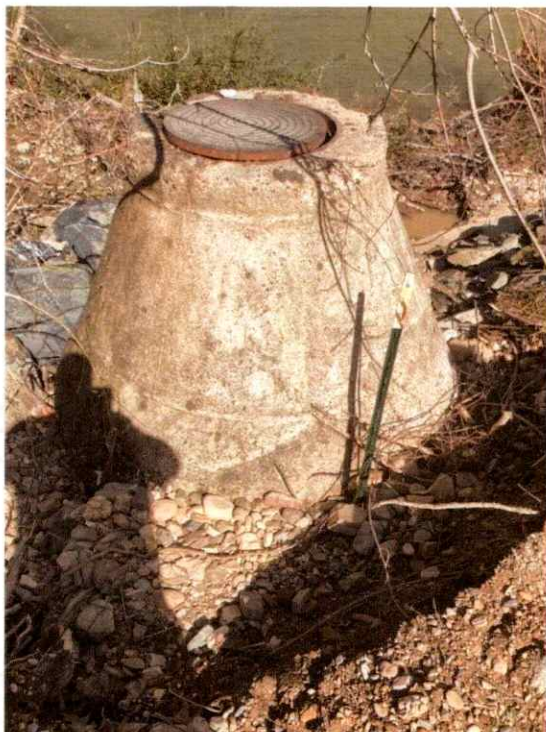
Manhole 1741 Before Cleanup
