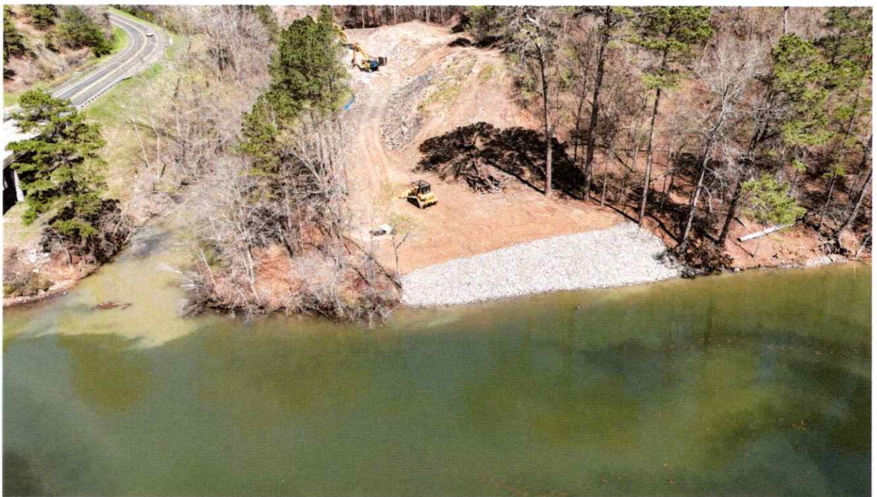
Davidson Drive WWTP Discharge
